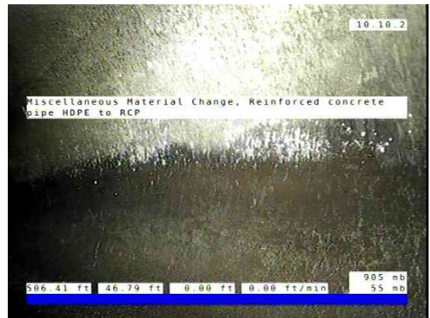
Inlet02-Inlet 03_3e24ec0e-4f99-405f-947d-06956c2e0b8c_20251010_0855 51_095.jpg, 00:03:08, 46.79ft Miscellaneous Material Change, Reinforced concrete pipe / HDPE to RCP
