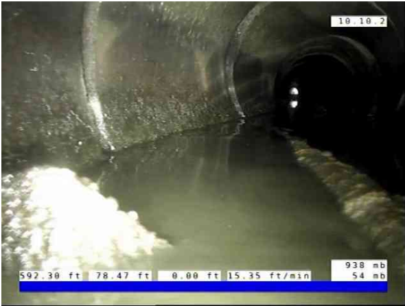
Inlet01-Inlet 02_ad0a5211-56df-4d64-bb13-9cbc7ff451ba_20251010_1419 01_282.jpg, 00:08:59, 78.46ft Deposits Settled Gravel, 5% of cross sectional area from 5 o'clock to 7 o'clock, within 8 inch, Finish
