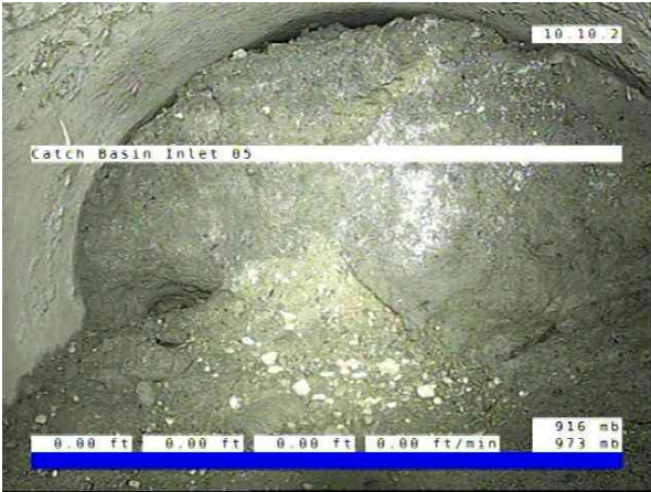
Inlet04-Inlet 05_770bcdde-84b8-4ac9-98a4-e624e9c8505c_20251010_100 716_451.jpg, 00:00:00, 0.00ft Catch Basin / Inlet 05
