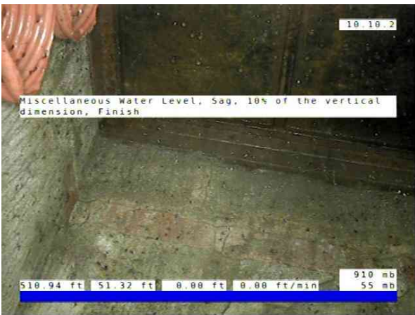
Inlet02-Inlet 03_b95ad3d4-e88c-4833-9959-994b44d98212_20251010_085 759_394.jpg, 00:04:40, 51.32ft Miscellaneous Water Level, Sag, 10% of the vertical dimension, Finish
