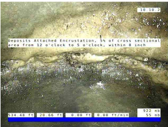
Inlet01-Inlet 02_e20c1c36-448b-4eb5-b83c-9f6c7296de66_20251010_090 334_265.jpg, 00:02:40, 20.66ft Deposits Attached Encrustation, 5% of cross sectional area from 12 o'clock to 5 o'clock, within 8 inch
