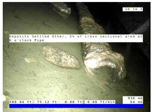
Inlet01-Inlet 02_d1fadcf8-0bdb-4cb0-9ea1-e30796fcc8aa_20251010_090945_947.jpg, 00:07:37, 75.10ft Deposits Settled Other, 5% of cross sectional area at 6 o'clock / Pipe
