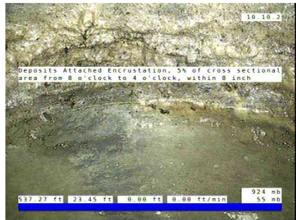
Inlet01-Inlet 02_5a08e344-e137-4ace-adff-32d12ace4808_20251010_0904 10_146.jpg, 00:03:05, 23.45ft Deposits Attached Encrustation, 5% of cross sectional area from 8 o'clock to 4 o'clock, within 8 inch
