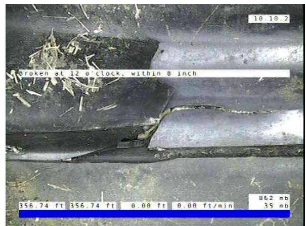
Inlet03-Inlet 04_e6c106fa-ce9d-409c-b7eb-d8a09dee563b_20251010_084 311_167.jpg, 00:14:47, 356.74ft Broken at 12 o'clock, within 8 inch
