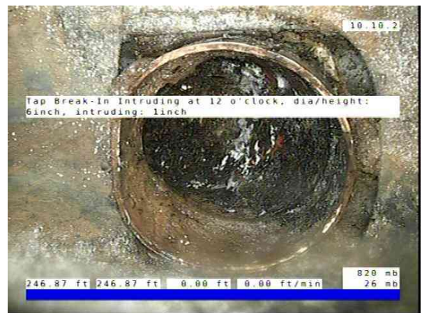
Inlet03-Inlet 04_e4ceac8e-e1ce-4ae5-bc7d-48c141ca7f75_20251010_0832 38_056.jpg, 00:09:52, 246.87ft Tap Break-In Intruding at 12 o'clock, dia/height: 6inch, intruding: 1inch
