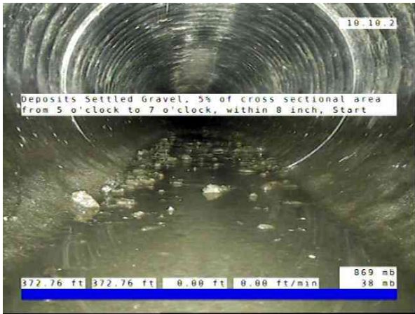
Inlet03-Inlet 04_ab22c8df-7f35-4172-bfd6-4f8122662604_20251010_084500_792.jpg, 00:16:12, 372.76ft Deposits Settled Gravel, 5% of cross sectional area from 5 o'clock to 7 o'clock, within 8 inch, Start
