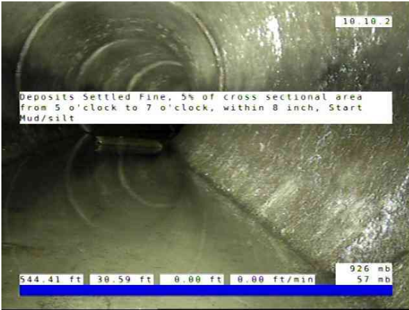
Inlet01-Inlet 02_78bf45a-64ba-49b3-9b29-682460321246_20251010_090502_970.jpg, 00:03:45, 30.59ft Deposits Settled Fine, 5% of cross sectional area from 5 o'clock to 7 o'clock, within 8 inch, Start / Mud/silt
