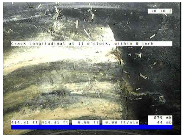
Inlet03-Inlet 04_d4728e8b-59c1-45ec-acbb-4fb24ba5e040_20251010_084748_747.jpg, 00:18:36, 414.31ft Crack Longitudinal at 11 o'clock, within 8 inch
