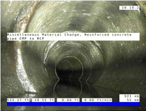
Inlet01-Inlet 02_5e12a33c-8def-4af7-947d-3fb8f3a82718_20251010_0902 51_999.jpg, 00:02:14, 19.55ft Miscellaneous Material Change, Reinforced concrete pipe / CMP to RCP
