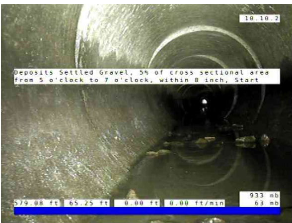
Inlet01-Inlet 02_2e7807ff-4cc5-4ebe-9fe1-969bbc6623a5_20251010_090826_600.jpg, 00:06:29, 65.25ft Deposits Settled Gravel, 5% of cross sectional area from 5 o'clock to 7 o'clock, within 8 inch, Start
