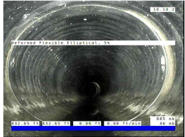
Inlet03-Inlet 04_7b49c65a-3867-4ab5-b404-749a917ac628_20251010_084 920_317.jpg, 00:19:44, 432.65ft Deformed Flexible Elliptical, 5%
