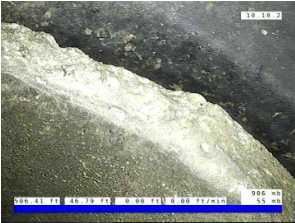
Inlet02-Inlet 03_27a9f95b-5a43-46f0-9739-0911ed2e6077_20251010_085 624_226.jpg, 00:03:11, 46.79ft Miscellaneous Shape or Size Change / 18" to 15"
