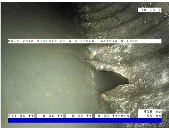
Inlet01-Inlet 02_6184eb40-fb5d-40c0-abf2-17b0dc0b82ab_20251010_0900 23_389.jpg, 00:00:27, 0.04ft Hole Void Visible at 4 o'clock, within 8 inch
