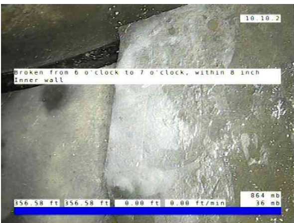
Inlet03-Inlet 04_2249918f-bb70-4c64-bd79-ce2412f1396b_20251010_0843 57_045.jpg, 00:15:21, 356.58ft Broken from 6 o'clock to 7 o'clock, within 8 inch / Inner wall
