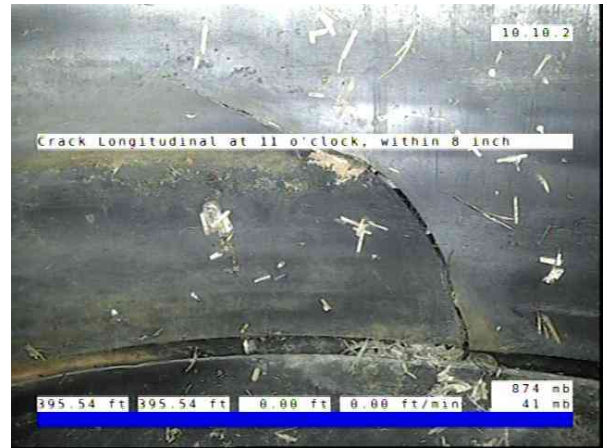
Inlet03-Inlet 04_1620e0c9-613f-49ce-823f-d7f66df169a2_20251010_084620_301.jpg, 00:17:23, 395.54ft Crack Longitudinal at 11 o'clock, within 8 inch
