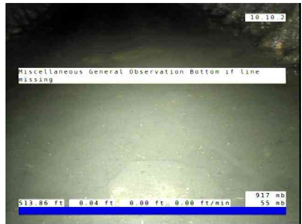
Inlet01-Inlet 02_1412f4ed-031a-452d-87f4-f99925acb638_20251010_0901 07_646.jpg, 00:00:42, 0.04ft Miscellaneous General Observation / Bottom if line missing
