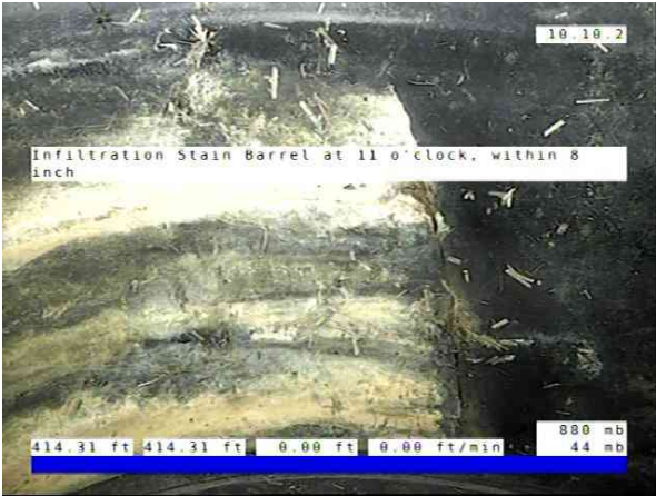
Inlet03-Inlet 04_e2809933-88e8-42e6-9239-637797dbe4f1_20251010_084 801_425.jpg, 00:18:41, 414.31ft Infiltration Stain Barrel at 11 o'clock, within 8 inch
