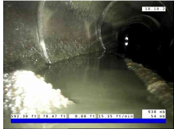
Inlet01-Inlet 02_d30c5ee5-1246-4ddc-a18a-74997edeaa6c_20251010_141 924_385.jpg, 00:08:59, 78.46ft Miscellaneous Survey Abandoned / Debris in line preventing further inspection
