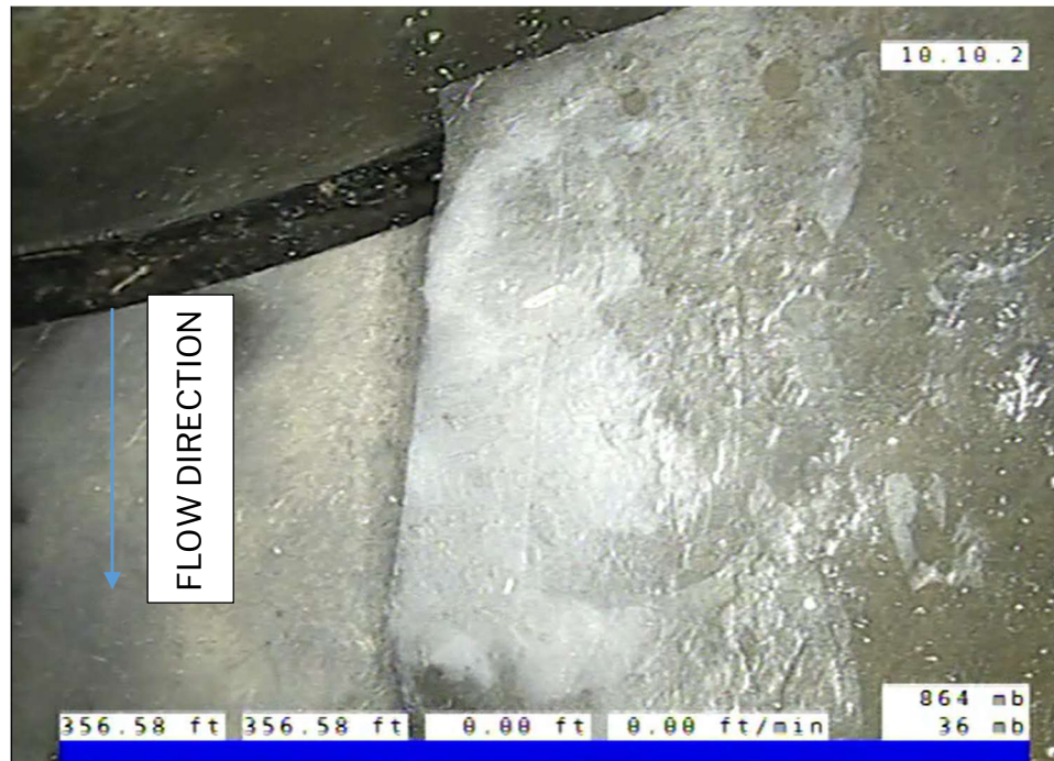
Figure 1: Broken Section of Pipe under Cherry Lane
