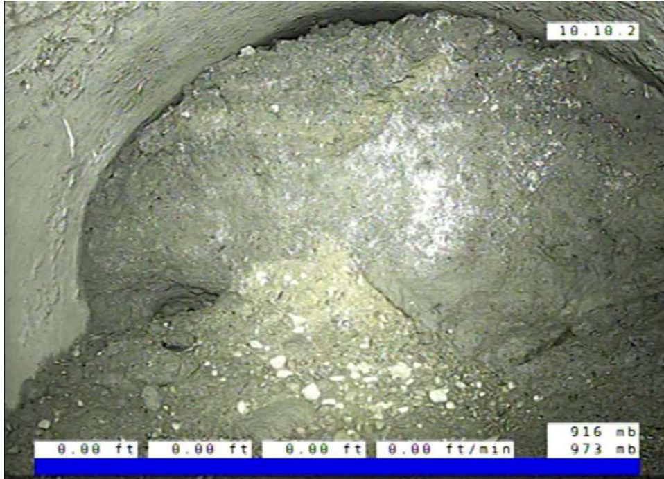
Figure 4: Blockage of storm sewer connection to the ODOT system at D8 (looking north towards D7)
