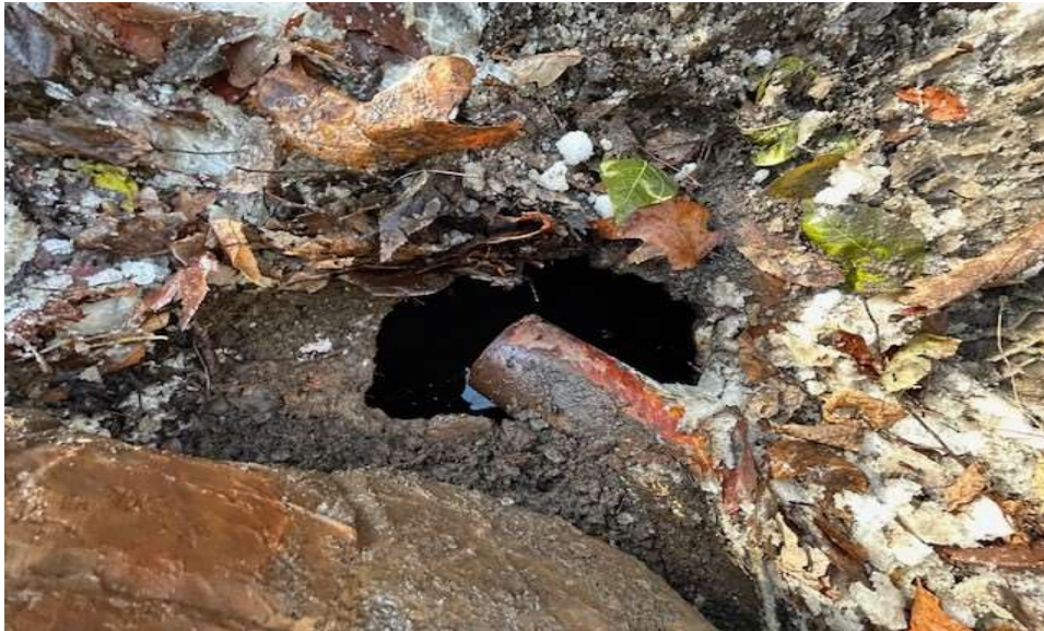
Figure 6: Gap in Pipe (denoted as Node D5), looking NW.
