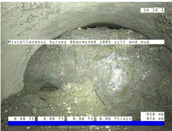
Inlet04-Inlet 05_0465d8d0-b35e-4f4c-983a-375dfc7bb184_20251010_1008 23_878.jpg, 00:00:44, 0.00ft Miscellaneous Survey Abandoned / 100% silt and mud
