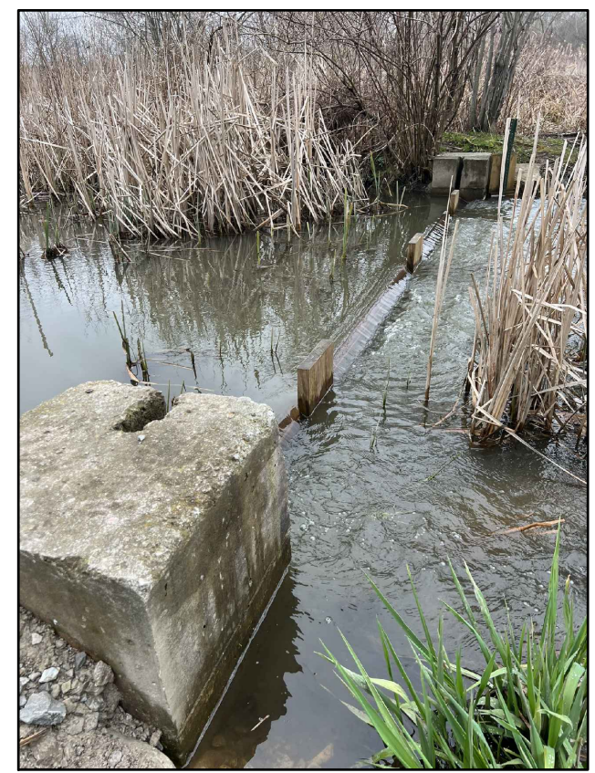
OUTLET CONTROL STRUCTURE PHOTO #2
