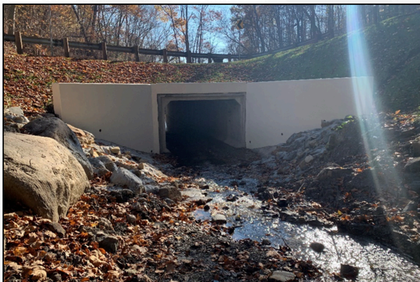
Bridge No. BAT-114-0320 N. Revere Road over Revere Run includes a new concrete box culvert structure, looking at the inlet end of structure.
