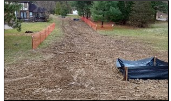
Replacement of storm sewer and overflow swale grading for Wye Road Flood Mitigation and Drainage Improvement Phase 1
