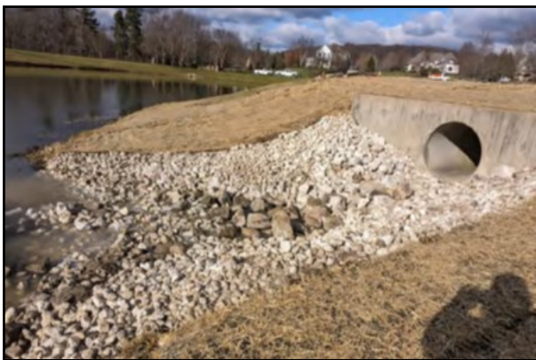
Repair of erosion at storm sewer outlet to retention pond in Firestone Trace
