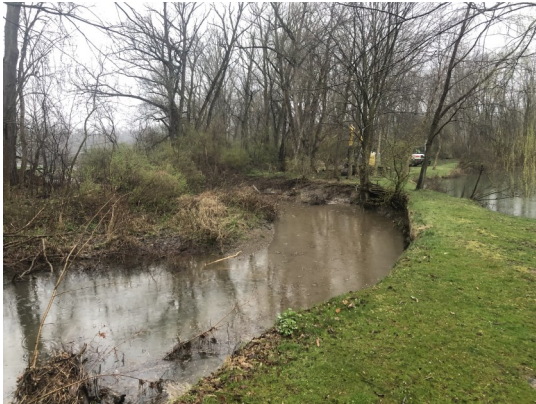
Streambank erosion was threatening to drain the retention pond in the Arbour Green subdivision.
