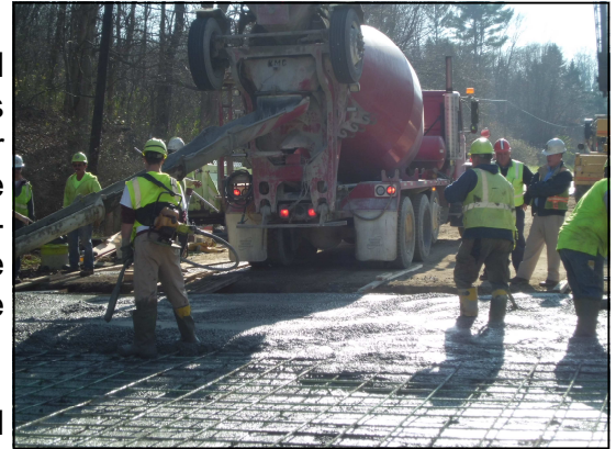
Workers pour concrete for the new deck on the Akron Peninsula Road Bridge
