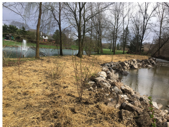
Photograph 6 (April 9, 2020). Shrubs, live stakes, seed, and straw were installed along the restoration area.
