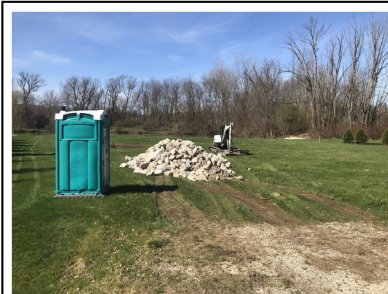
Photograph 1 (April 6, 2020). Stone, an excavator and sanitation facilities were brought to the site.
