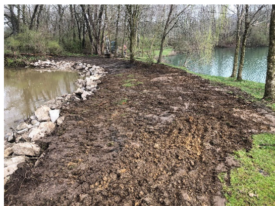
Photograph 4 (April 9, 2020). Onsite material was backfilled into the intervening space adjacent to the toe protection and the stream bank was regraded to a stable slope. The causeway between the stream and the pond has been extended 10 to 12 feet.
