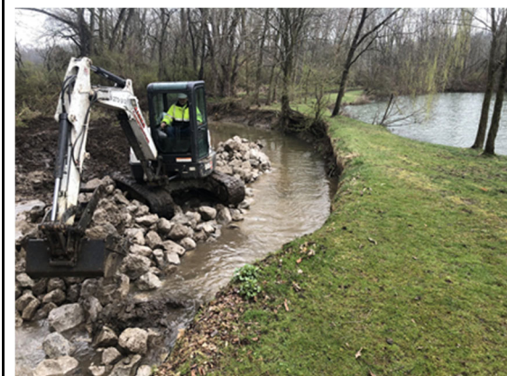
Photograph 3 (April 8, 2020). Toe protection was installed in the stream. The intervening area between the toe protection and the eroded bank was backfilled.
