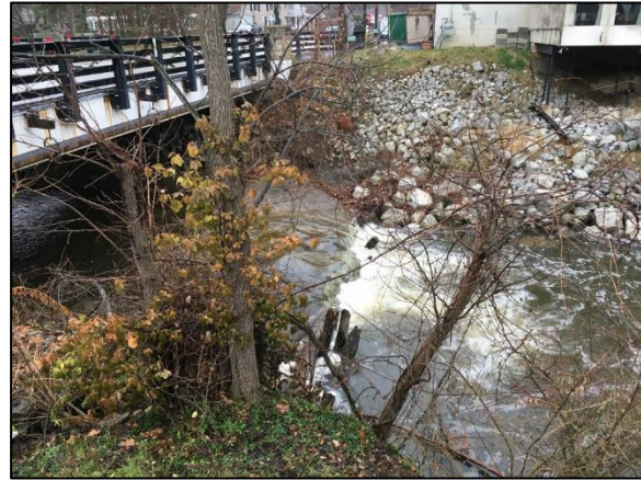
Figure 42: Scour hole downstream of bridge and rock protection along Lanning's
