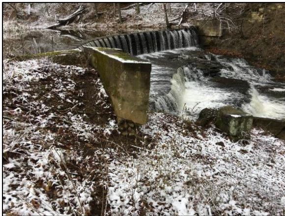
Figure 65: Right abutment is leaning with a home under construction downstream.
