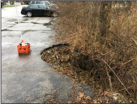
Figure 41: Erosion in parking lot creating safety issue for users
