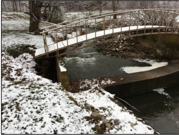
Figure 8: Private bridge with tall, unstable banks and flanking behind bridge abutments
