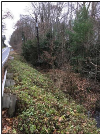
Figure 73: Leaning power pole
