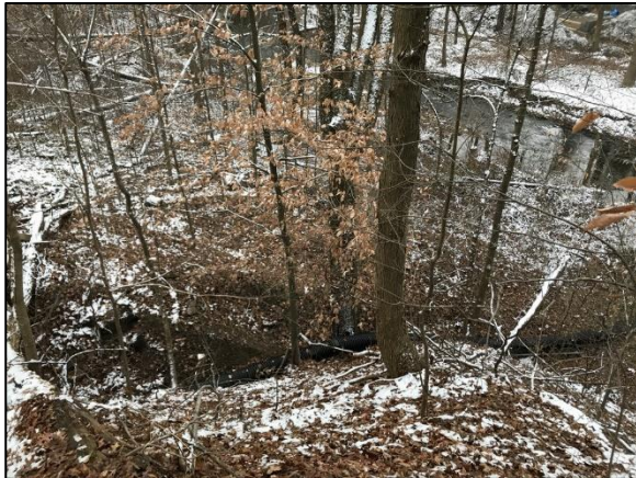
Figure 20: Black HDPE pipe lying in the ravine with Yellow Creek in the background
