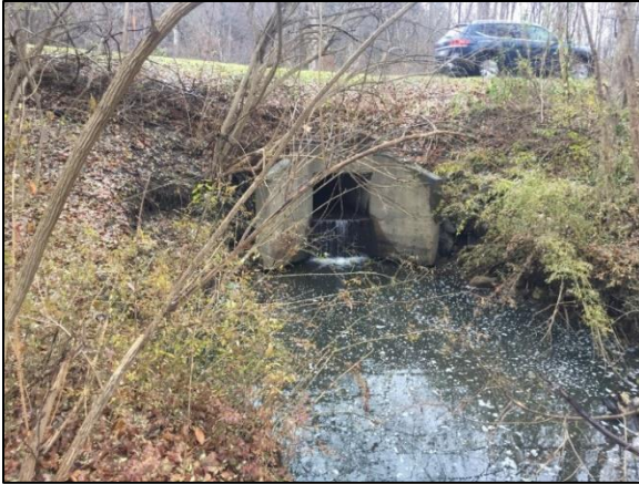
Figure 63: Culvert outfall with large scour pool that potentially risks exposing and/or undermining the culvert
