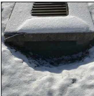
Figure 19: Erosion at inlet
