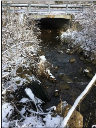
Figure 69: Exposed geotextile in the foreground
