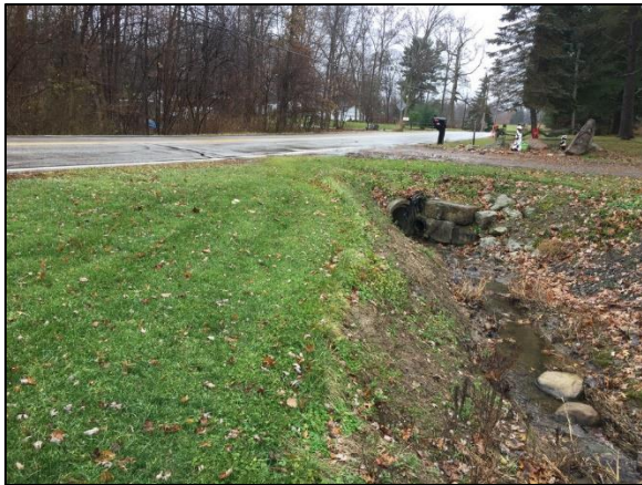
Figure 17: Culvert under Revere Road reported to have overtopped during past rain events
