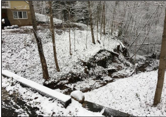
Figure 37: Eroded ravine downstream of driveway
