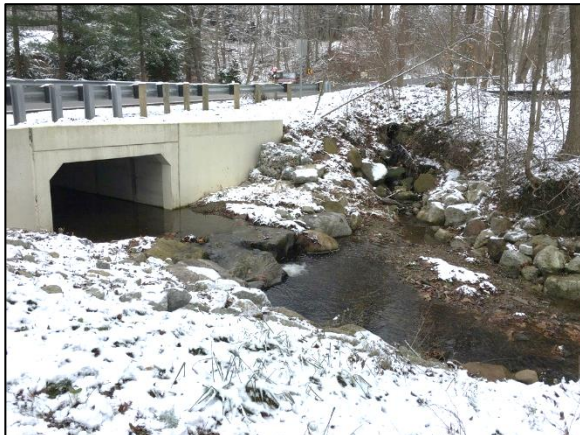
Figure 18: Eroded stormwater outfall next to bridge
