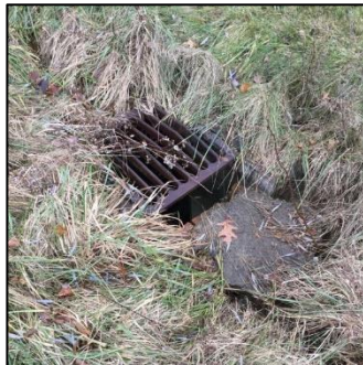
Figure 16: Erosion and concrete failure at inlet
