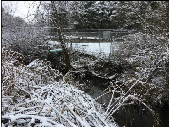
Figure 46: Exposed pipes in bank show extents of bank erosion along WWTP fence
