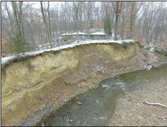
Figure 4: Geotechnical mass wasting (bank failure) along Lower Yellow Creek.
