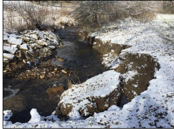
Figure 61: ~6-foot slump in residential backyard lacking riparian vegetation.
