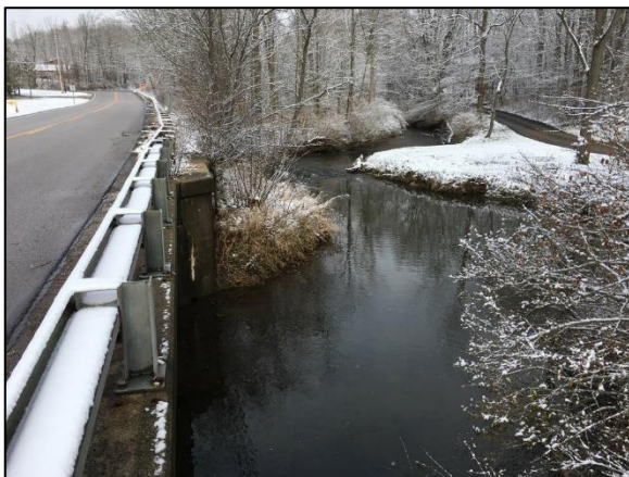
Figure 40: Yellow Creek along Crystal Lake Road, looking downstream at alignment and erosion
