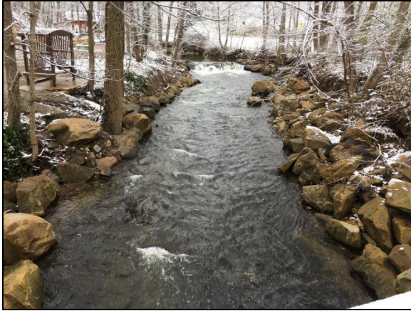
Figure 60: Loose rock bank protection on a private property
