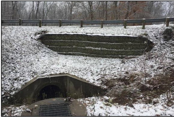
Figure 67: Slumping gabions along Bonnebrook Dr.
