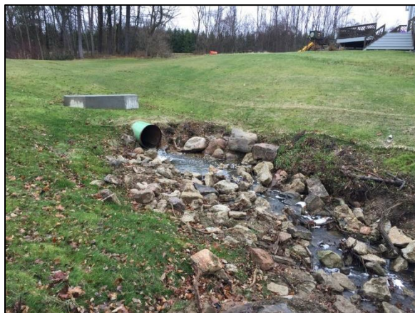
Figure 43: Bare bank areas downstream from the outfall indicate mobilized armoring
