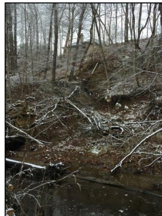
Figure 51: Major erosion and mass wasting at pipe outfall
