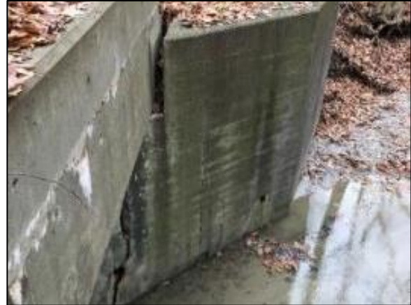
Figure 64: Cracked bridge abutments
