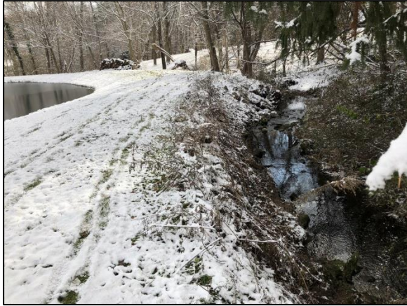
Figure 48: Basin embankment with erosion on the bank of West Creek
