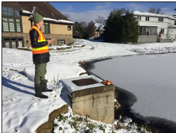
Figure 22: Outlet control structure at Arbour Green South basin
