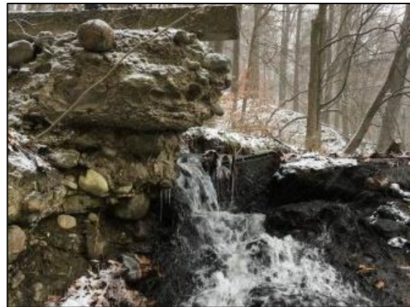
Figure 66: Dam is patched with a piece of plywood & chain-link fence.
