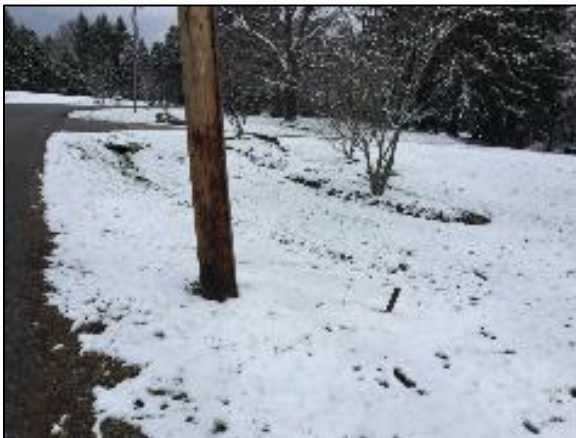
Figure 33: Culvert along Ranchwood that directs flows onto driveway at 4826 Ranchwood
