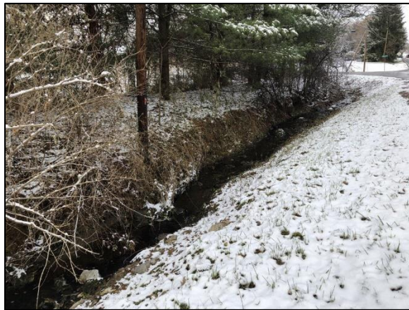
Figure 70: Eroded channel with partially exposed power pole
