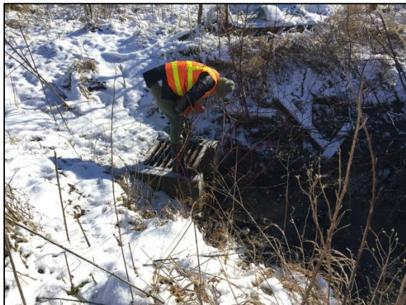
Figure 21: Outlet control structure at Arbour Green North basin
