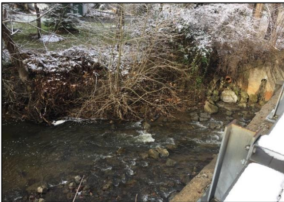
Figure 68: Bank erosion downstream of bridge
