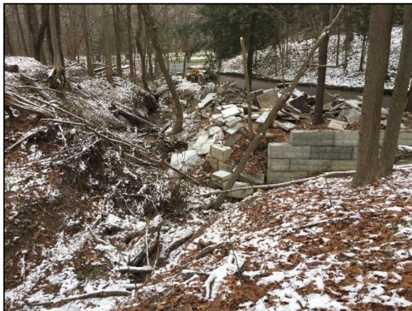
Figure 30: Confluence of tributaries with mass wasting and compromised retaining walls
