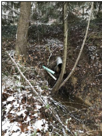
Figure 36: Undercut stormwater pipes document erosion in ravine
